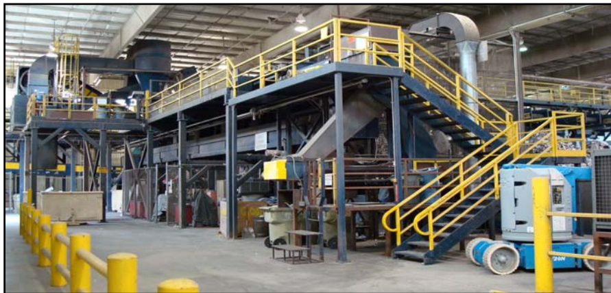
Materials Recovery Facility
