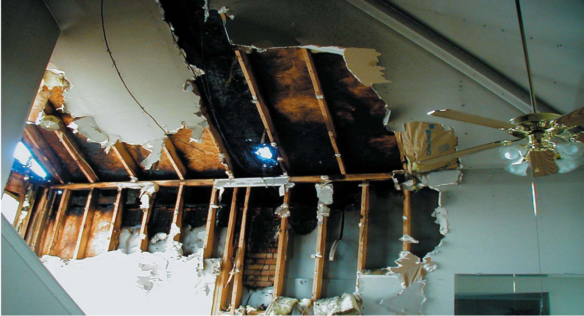
Water damaged building inspected by Building Safety
